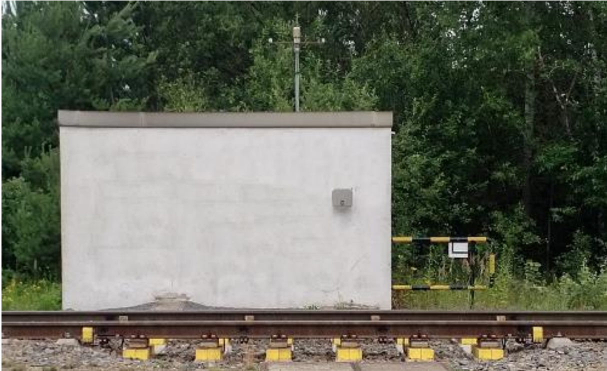
Fig. 2: RFID antenna on the track
